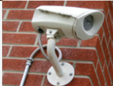
Home Security & Biometric Access Control Systems
